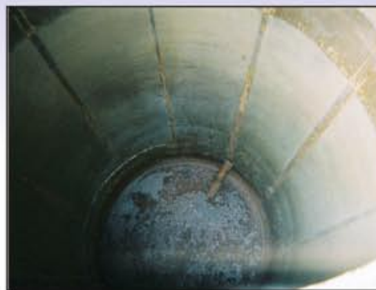
Interior Of Chemical Storage Tank Displaying Wear
